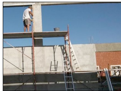
Expansion continues on Dodoma Innovation & Production Company's (DIPC) water bottling plant. This separate, for-profit business is committed to helping support DCMC.
